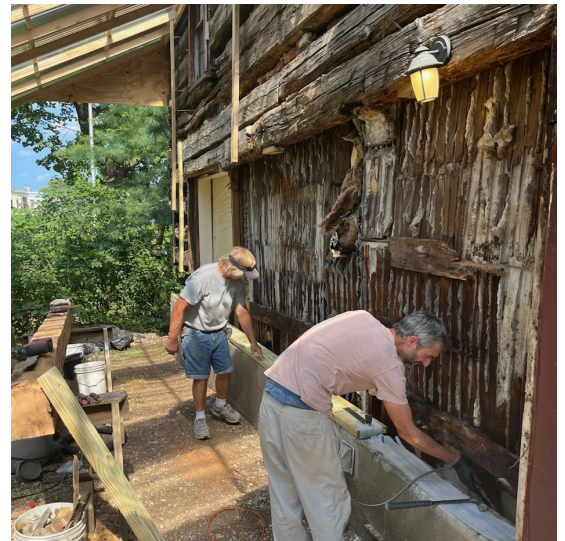
Contractor Frank Stroik (left) installs a new sill after removing deteriorated logs, while Stenton Site Manager Jeff Eckel treats the interior wall for insects.
